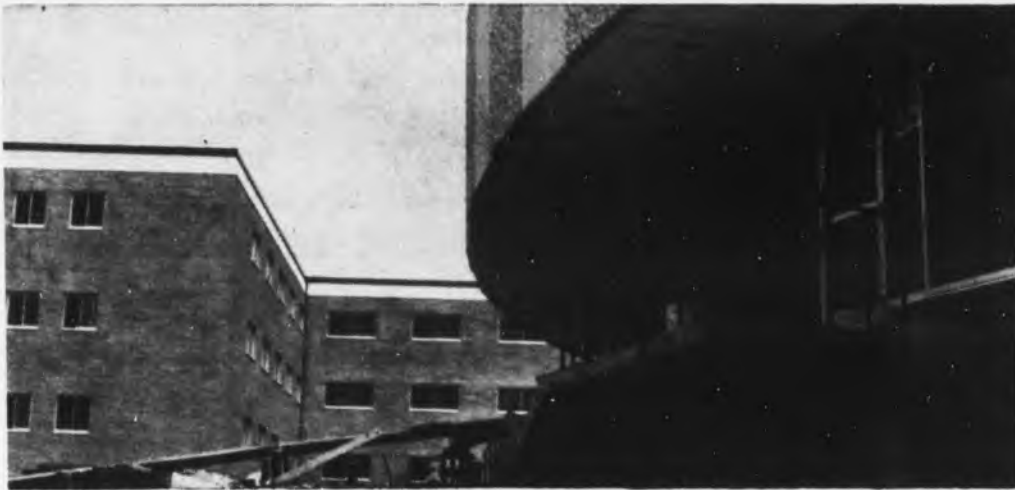
CONSTRUCTION PROGRESS SHOT —Construction work of the new dormitory nears completion for occupancy in September. The picture here shows one of the four living areas to the left and to the right the circular dining and main lounge area. Each living complex will have a separate lounge also. See story on page 1.
