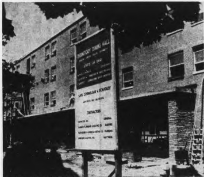
THE NEW DINING HALL, located on the site of the old commons will serve 1,200 students. Pictured is the loading dock on the north side of the building.
