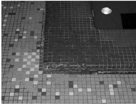
Figure 7 — Broken tiles on pool deck.
