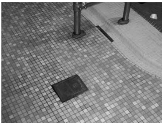
Figure 4 — Rusted drain cover.
