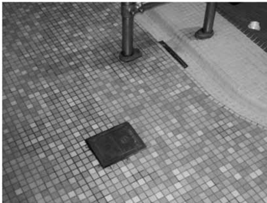
Figure 4 — Rusted drain cover.
