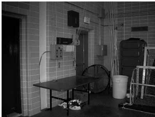
Figure 2 — Unorganized equipment blocking an exit.
