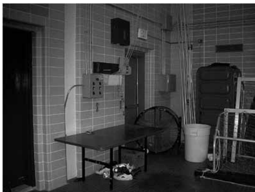
Figure 2 — Unorganized equipment blocking an exit.
